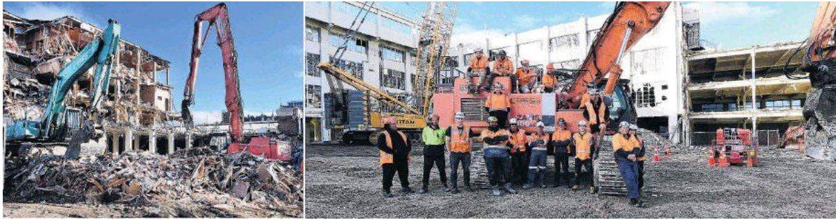
Wrecking crew . . . Ceres demolition plant matches the scale of the task as company staff survey the centre of the rapidly disappearing former Cadbury factory.
